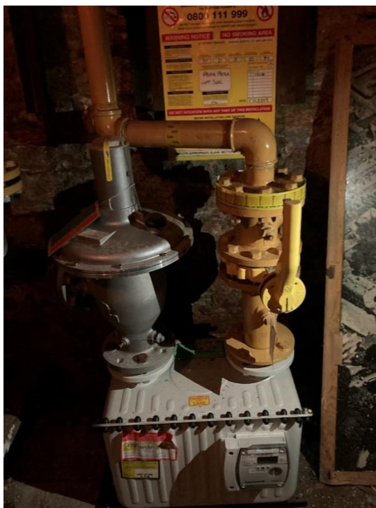
Figure 4 – Gas meter arrangement, 2” (DN50) pipework.
