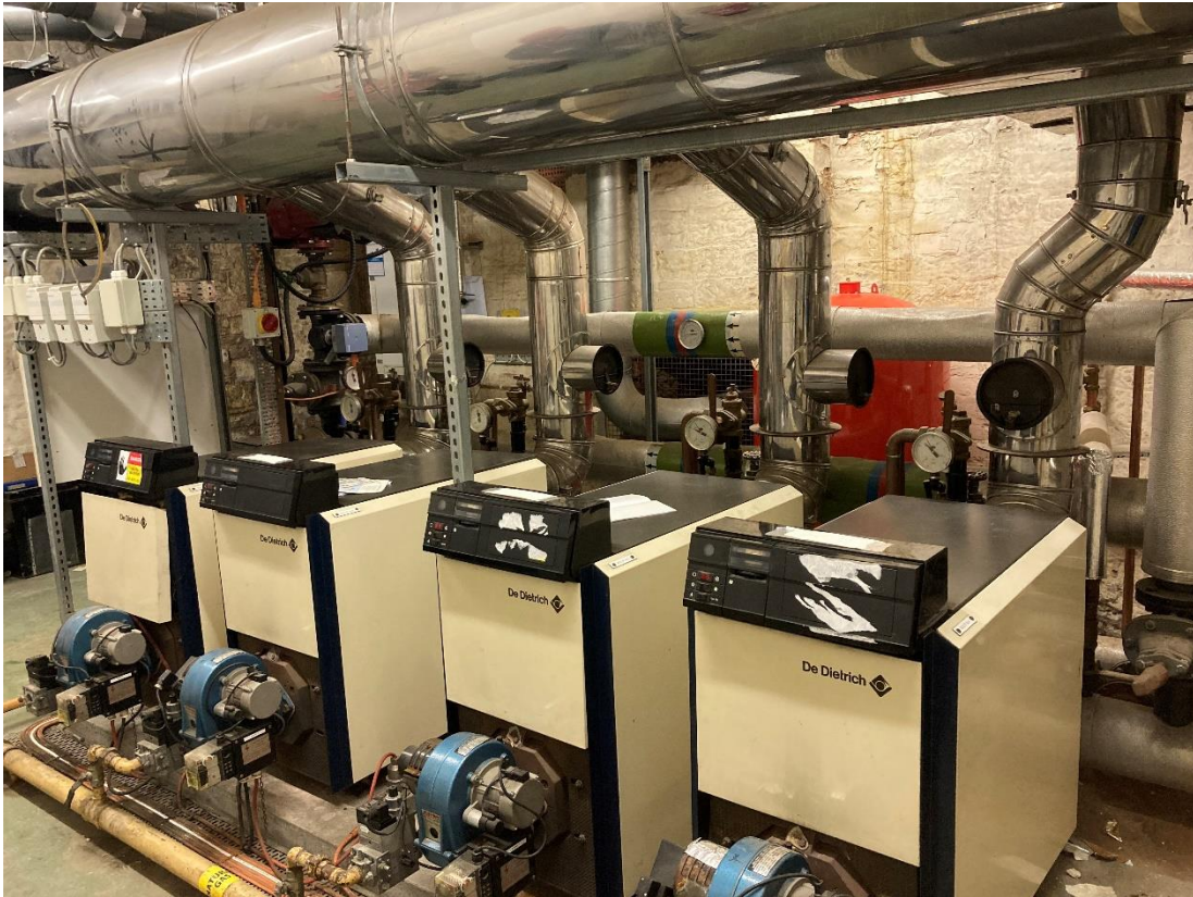
Figure 5 – Gas-fired boilers in the plantroom.
